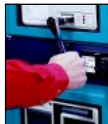
The drawout breaker can be conveniently racked in or out, stopping at the various positions with the door closed.
