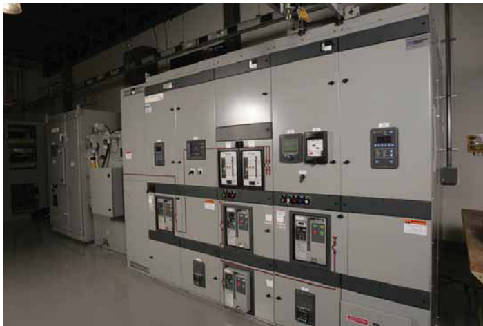
Low voltage switchgear
