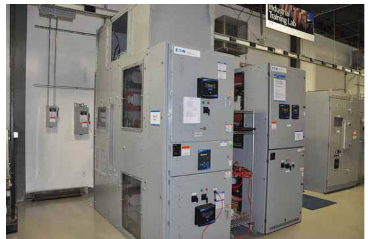
Medium voltage switchgear
