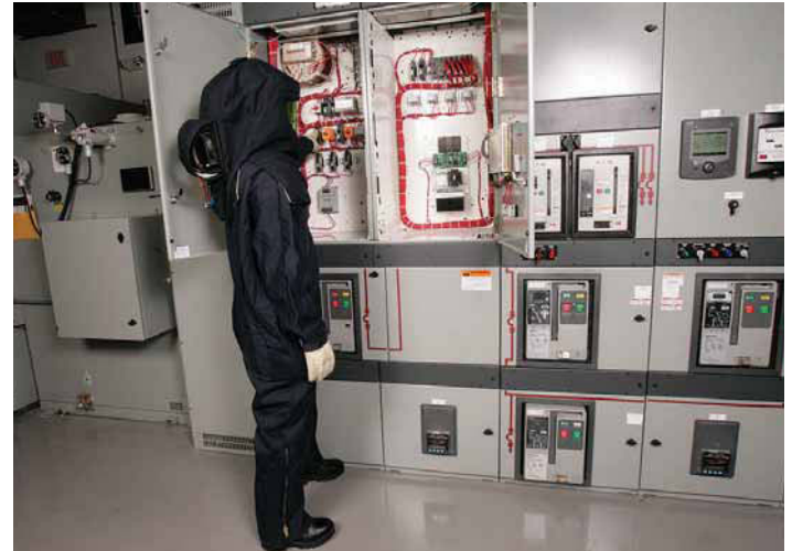
Worker wearing PPE inspecting low voltage switchgear
