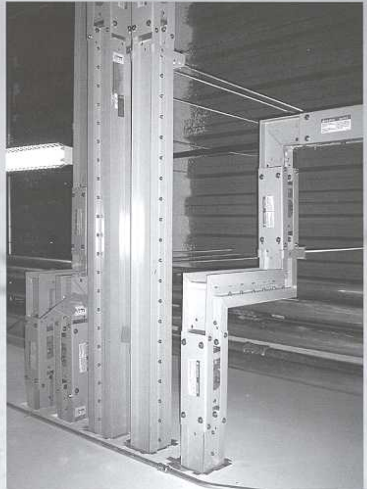
Typical busway installation
