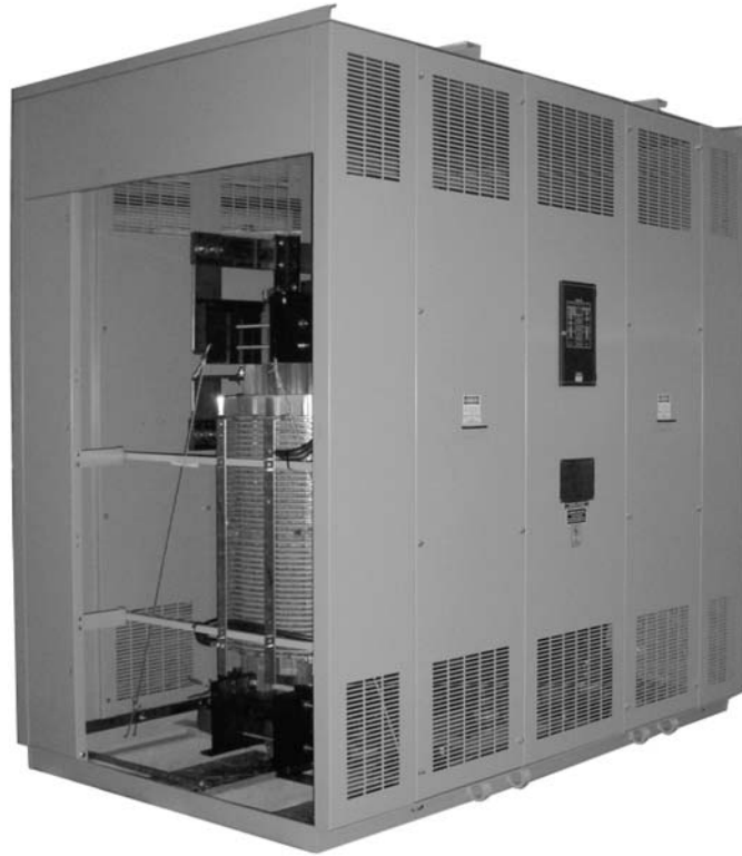
Dry-Type Unit Substation Transformer
