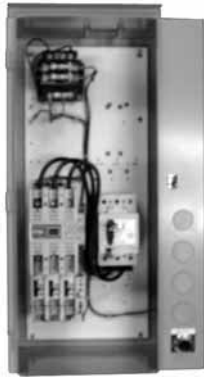
Irrigation Pump Panel
