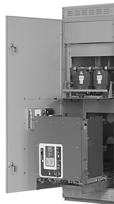
MEB Metal-Enclosed Switchgear
