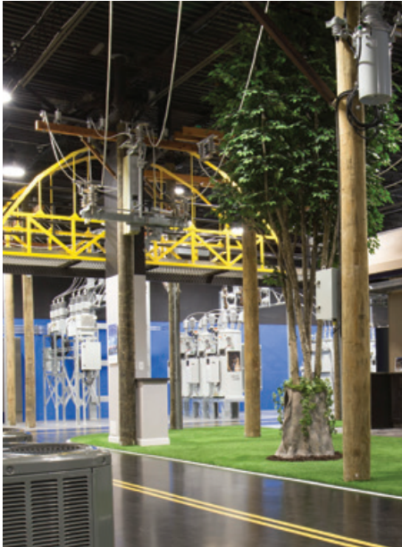
Utility substation and distribution
