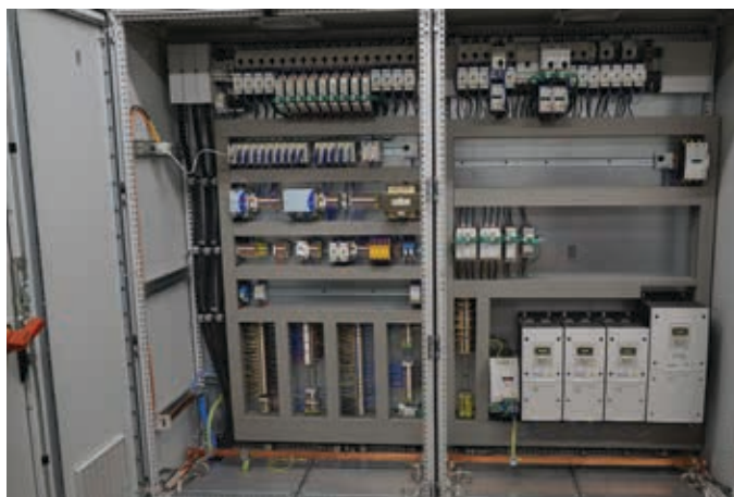
For the control and protection of the motor electronic motorstarters EMS and PKE are used. The drives of the conveyors between the stations are now frequency-controlled with the help of Eaton DA1 variable frequency drives.
