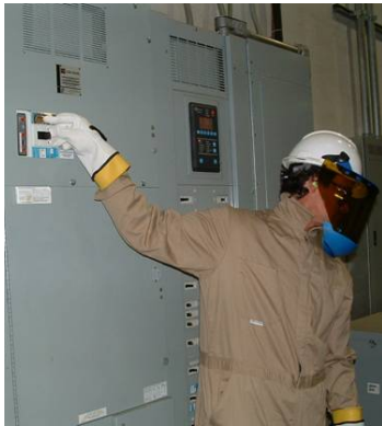
Figure 1. Bad Practice – Exposed Back of Neck
