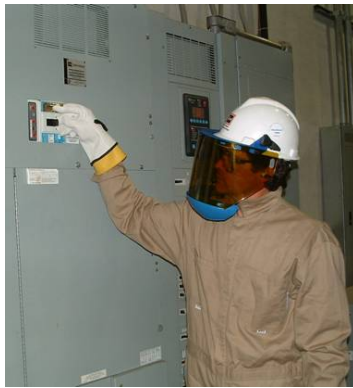
Figure 2. Good Practice – Entire Body Protected
