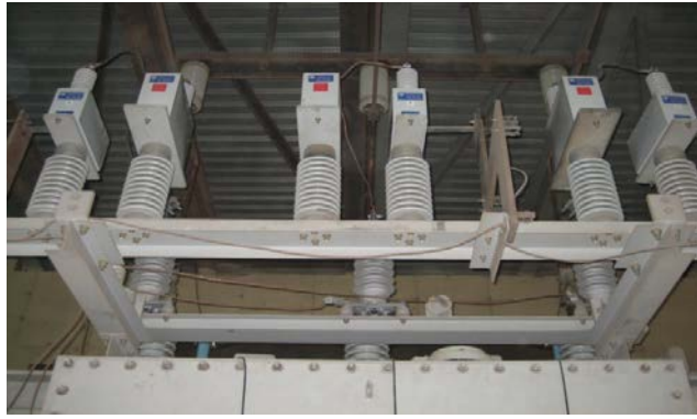
Figure 2. The surge arrester, capacitor and resistor removed for LMF1
