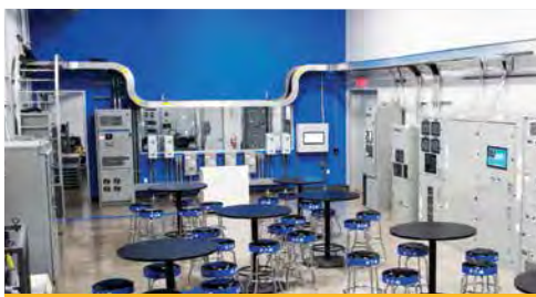
5. Power quality lab & motor room
