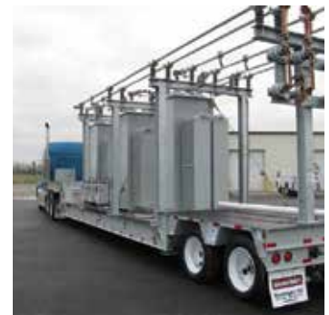
Modular Integrated Transportable Substations
