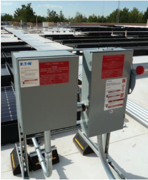
Eaton Solar Combiner Boxes
