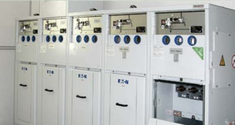
Compact: five panel Xiria E switchboard of the Alpstübli transformer station
