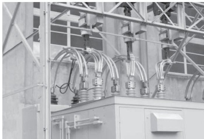
Figure 9. Circuit Breaker Bus Connections (Photo Courtesy of Southern Company)
