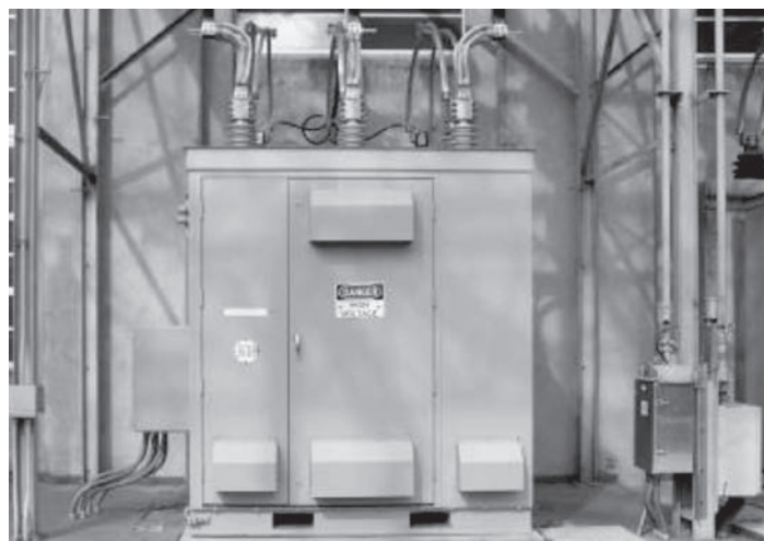
Figure 10. Installed Vacuum Circuit Breaker (Photo Courtesy of Southern Company)
