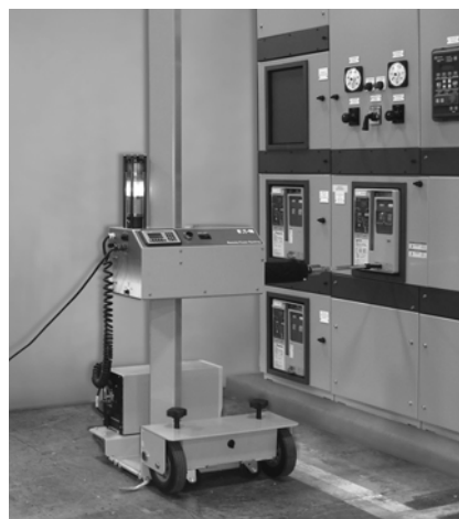
Remote Power Racking System
