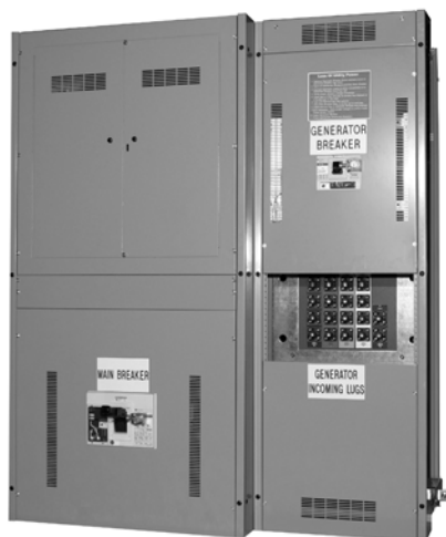
Generator Quick Connect Switchboard Section
