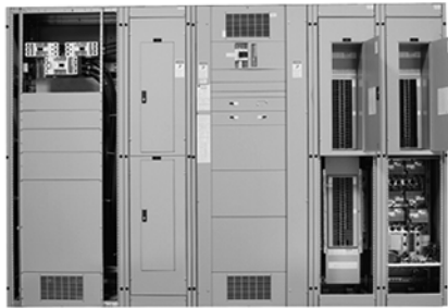
Integrated Facility System Switchboards
