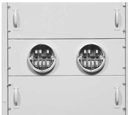
Meter Socket Sealable Cover Arrangement
