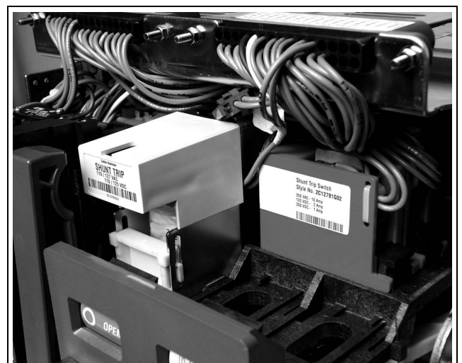
Figure 3-33: Shunt Trip Switch Installed
