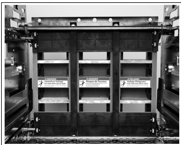
Figure 3-45: Safety Shutters in Open Position
