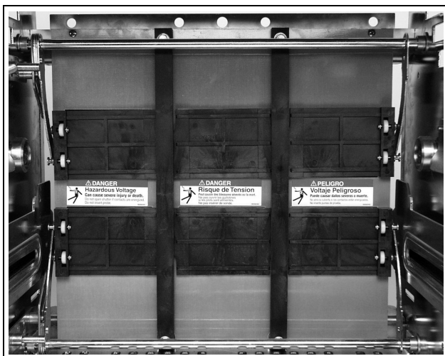
Figure 3-44: Safety Shutters in Closed Position
