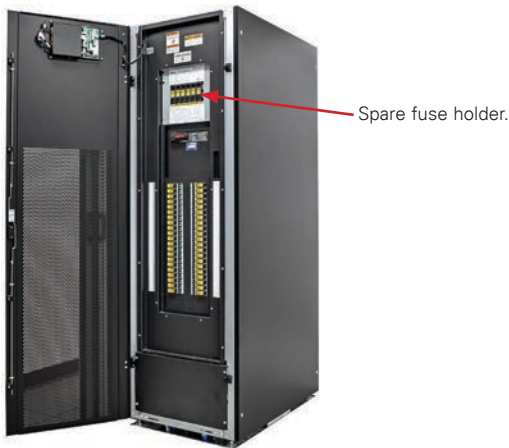
Figure 8.1.8.2.e RPP with QSCP chassis and spare CUBEFuse holder. Courtesy Liebert FDC— power distribution cabinet from Emerson Network Power™.
