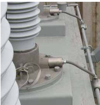
Sensor installed in capacitor tap of bushing
