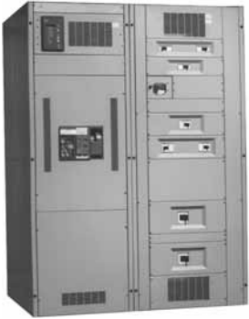
Front View—Circuit Breakers
