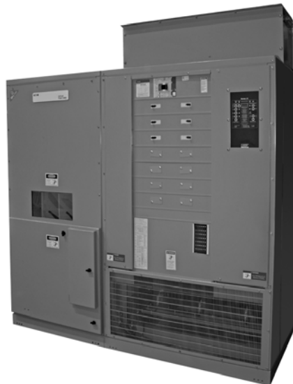
Unitized Power Center
