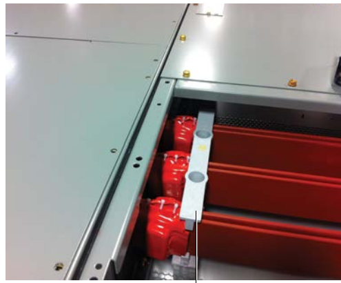
Main Bus Splice Between Unit Split
