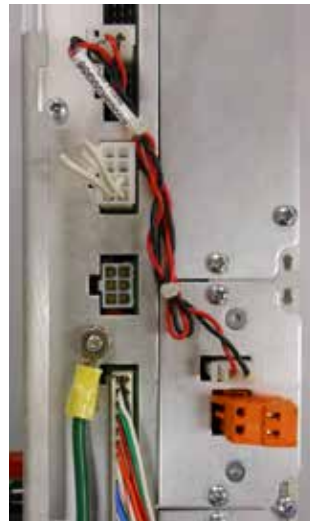
Figure 11. DC power module fully installed.
