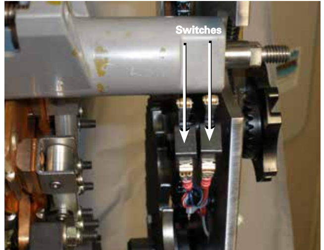
Figure 8. Loose logic switches.
