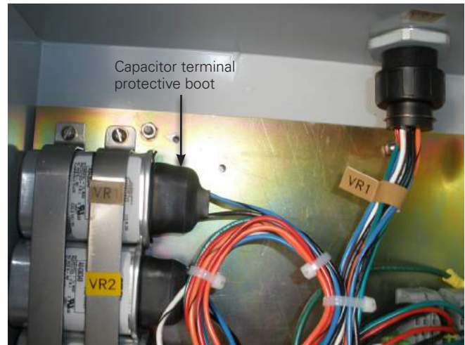
Figure 14. Capacitor protective boots.
