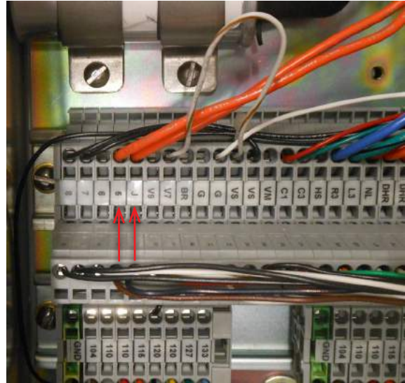
Figure 11. Orange wires shown relocated for VR1 and VR2. Each non-Cooper Power series connected voltage regulator requires relocation of an orange wire.
