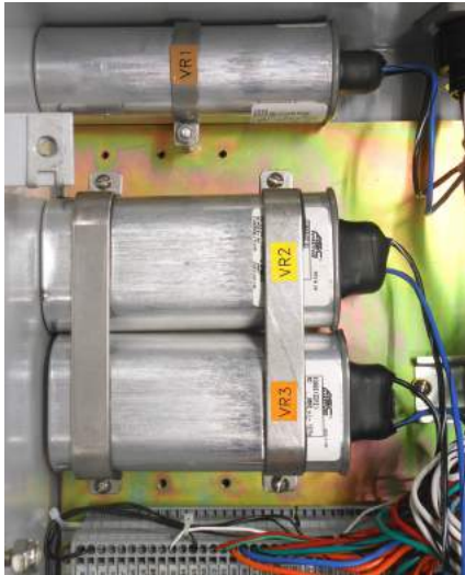
Figure 12. Multi-phase motor capacitor provisions.
