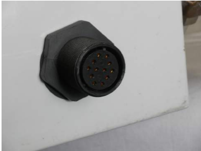
Figure 40. QCA connector coming from the bottom of the Siemens/Howard control box.
