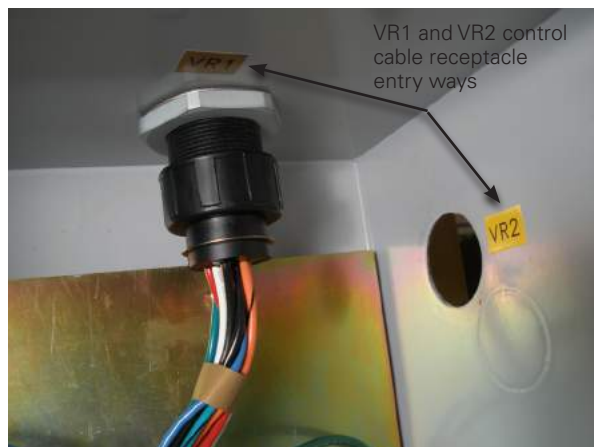
Figure 2. Enclosure entry way examples.
