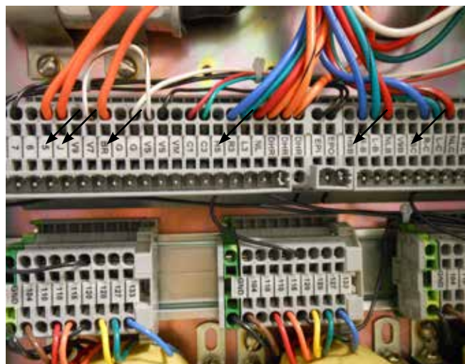
Figure 13. Orange wires moved from terminals HS, HSB, and HSC to terminals 5, J, and BR respectively.
