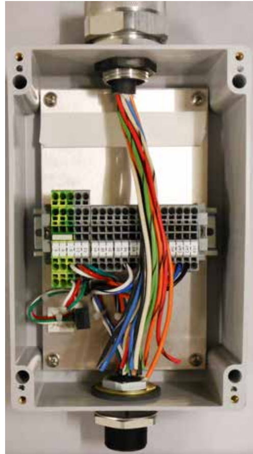
Figure 7. Control cable protruding into the junction box.
