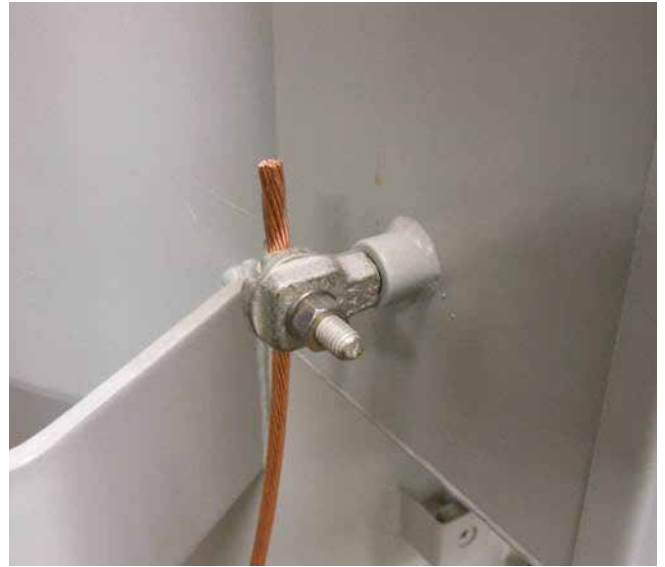
Figure 9. The control cabinet with ground cable connected.
