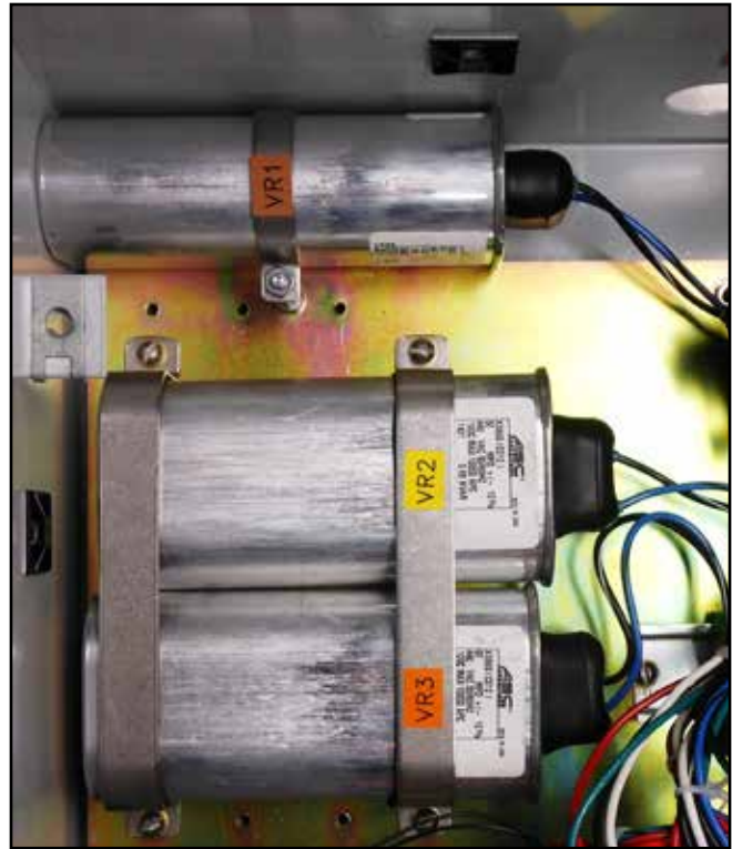
Figure 16. Another example of motor capacitor installation in a multi-phase voltage regulator control box.
