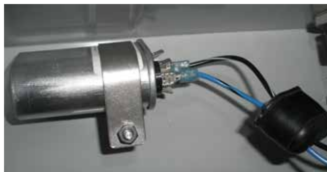
Figure 14. An example of motor capacitor installation in a single-phase voltage regulator control box.
