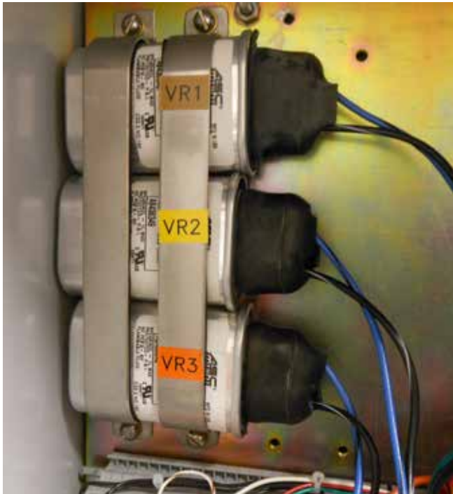
Figure 15. An example of motor capacitor installation in a multi-phase voltage regulator control box.
