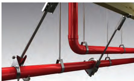
Branch line restraint
