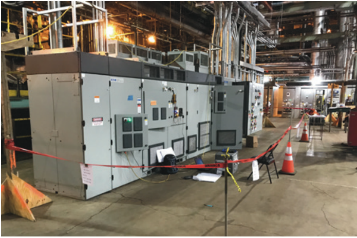
New medium-voltage drive and switchgear for starting package
