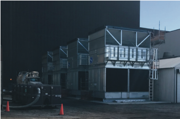
New closed loop hybrid cooling system
