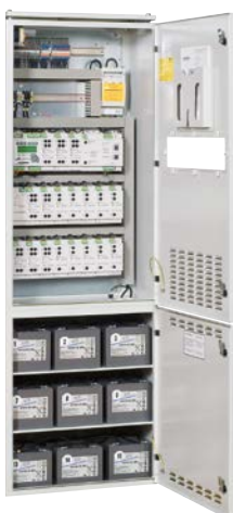
Non-hazardous area CEAG Emergency supply system
