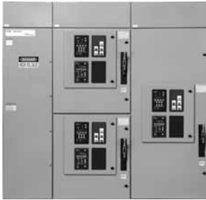
Next Generation AMPGARD Lineup— Front View
