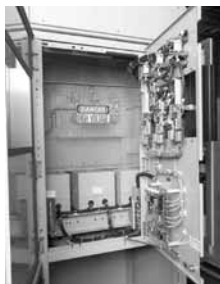
Mark V Field Controller
